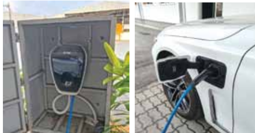
Electric Vehicle Charging Unit at our corporate office
